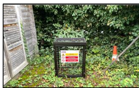
Gas Storage Cage
